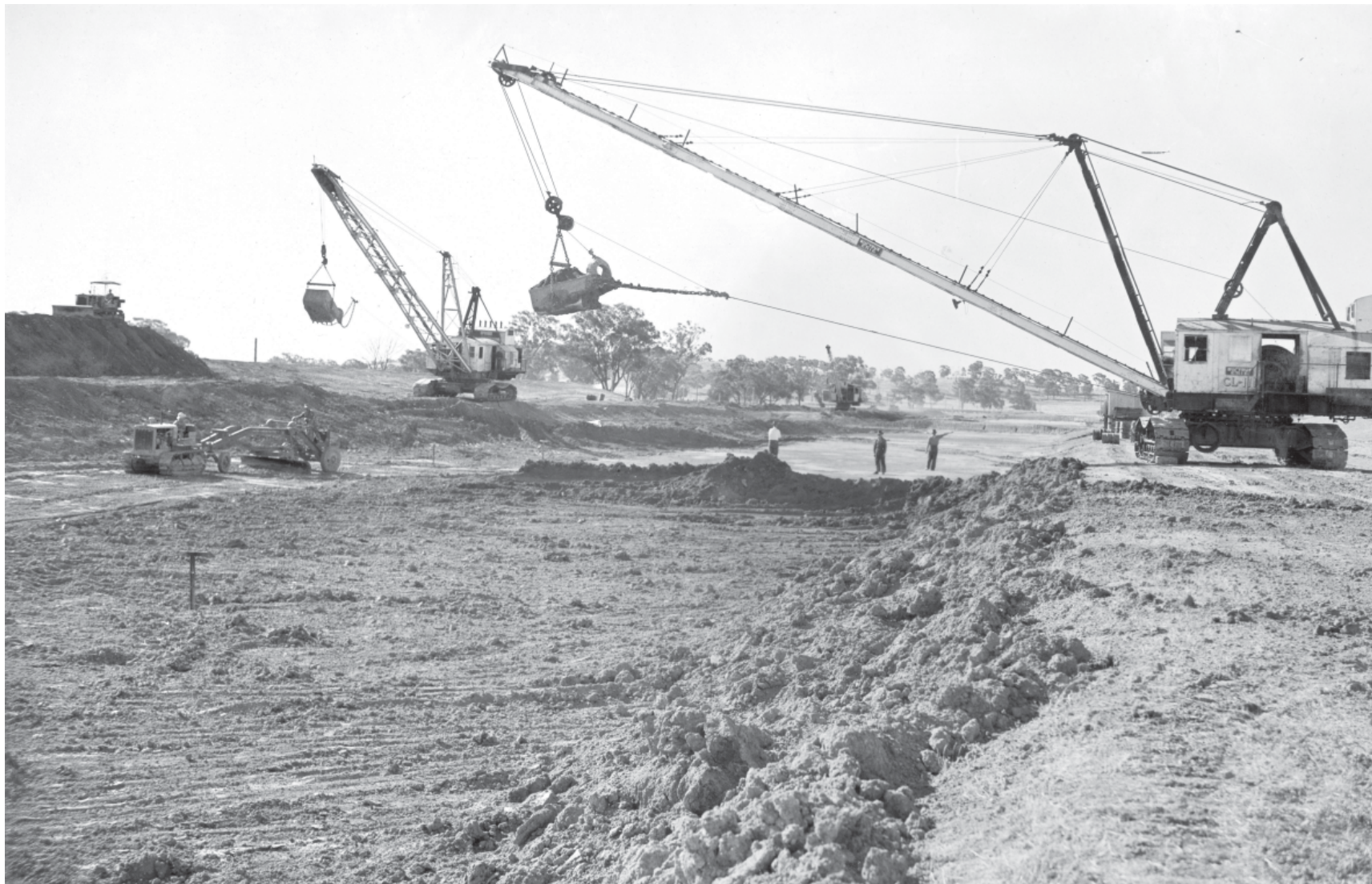
Bucyrus Erie dragline excavators were used in building the Mulwala Canal, Australia’s largest irrigation supply channel. Photo: State Water Archives Collection.
